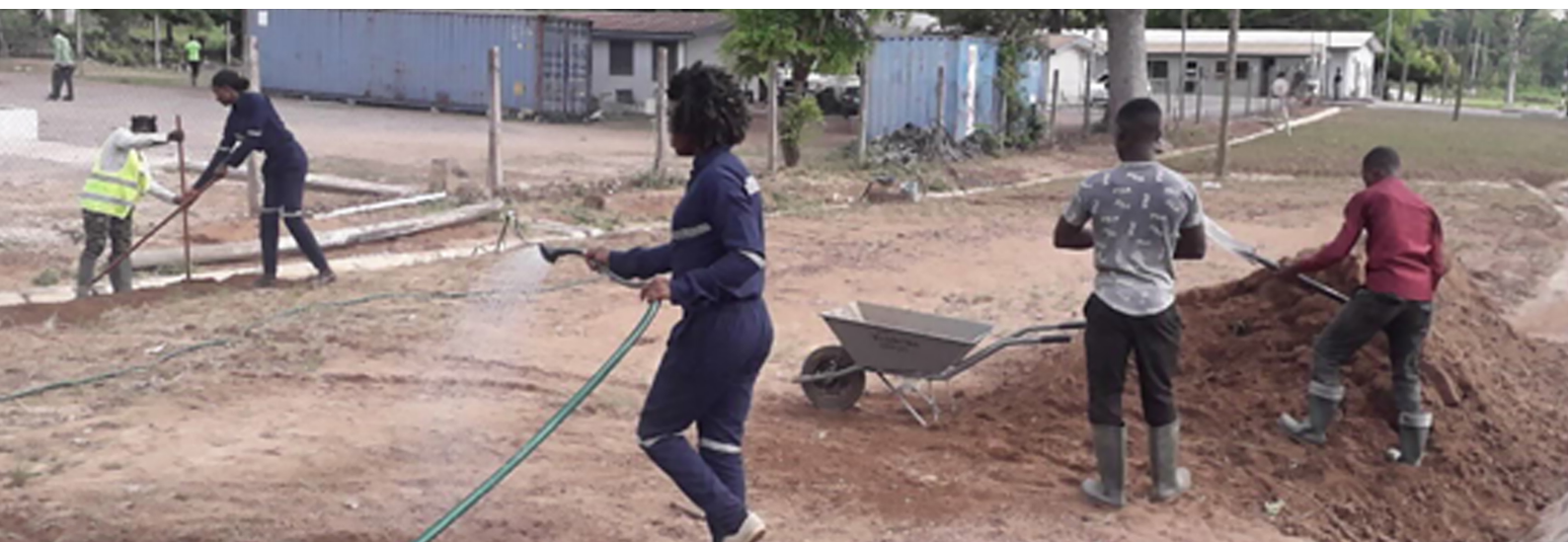
Management of Fire and Landscaping Group undertaking landscaping works at the project office area
