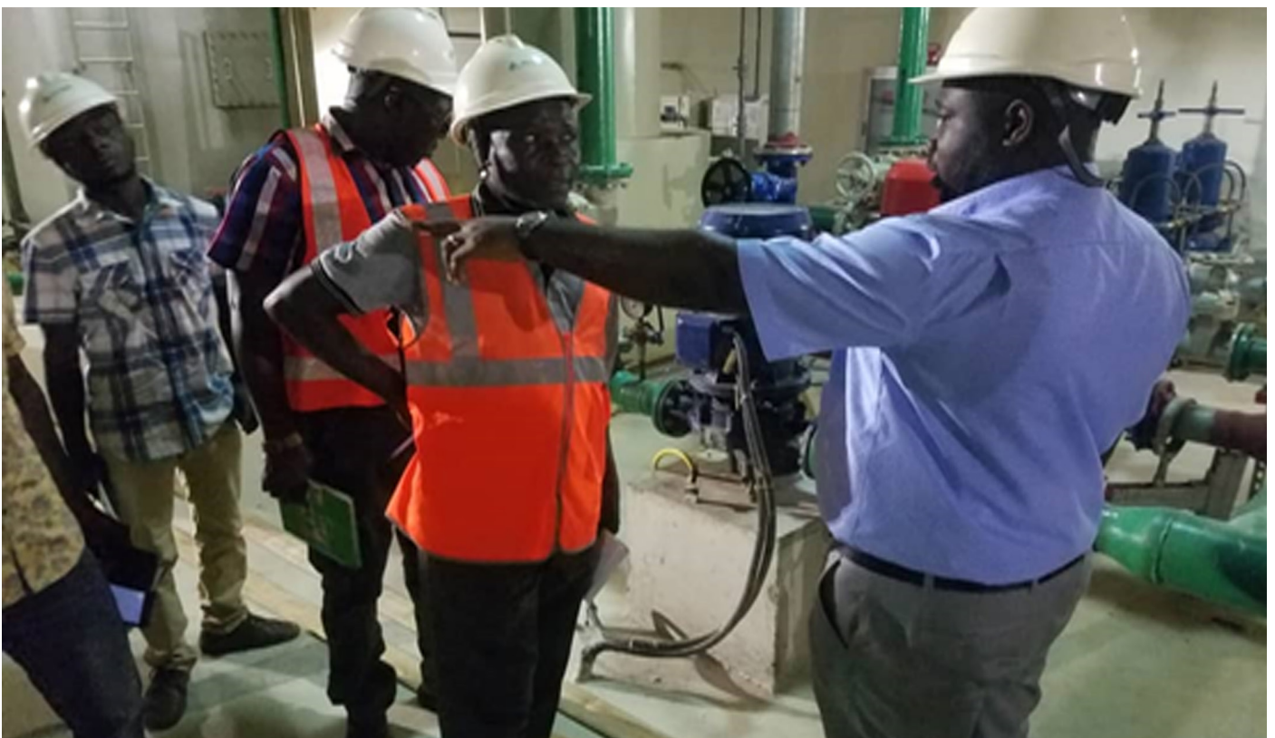
Department of Factories Inspectorate officials being briefed at BGS during an inspection
