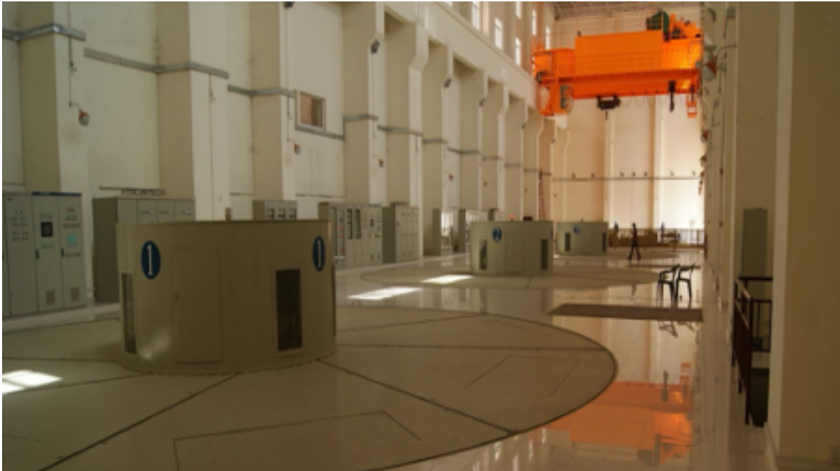
Figure 12. The generator floor showing the three Units (i.e., unit 1, unit2 and unit3)
