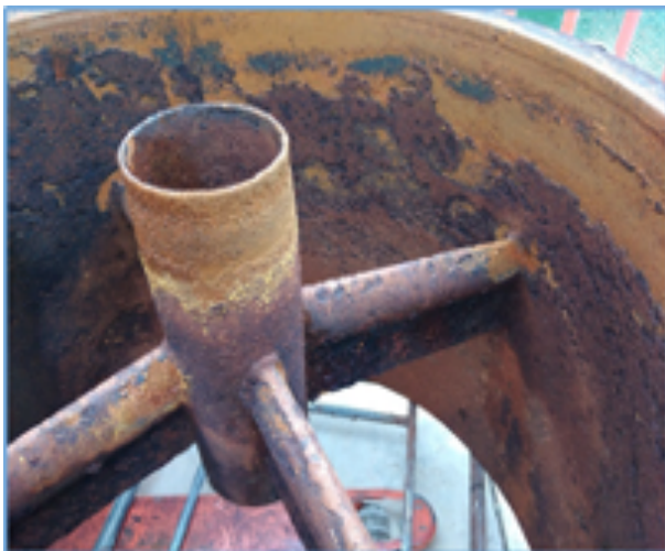
Figure 22: Air admission pipe (worn)
