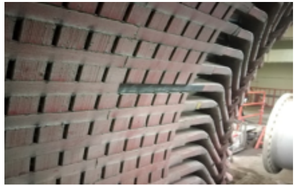
Figure 18: Stator wedge not in place
